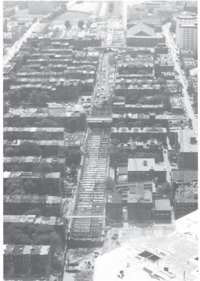
Fig. 4. The Southwest Corridor under construction literally illustrates the linking of abutting neighborhoods.
